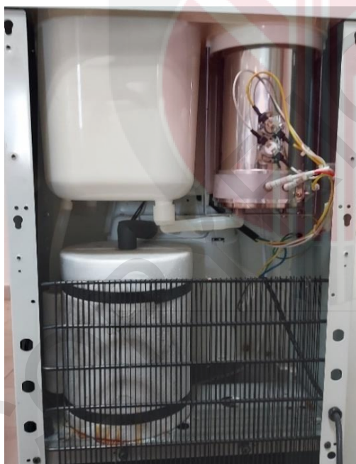
Figure 5.7: Plastic parts in water filter machine J
