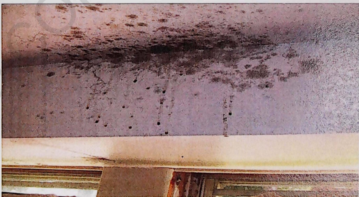
Figure 1.2 Mold problems on ceiling
