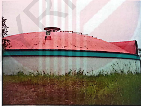
Figure B2: Reservoir water tank UPMKB (S2)
