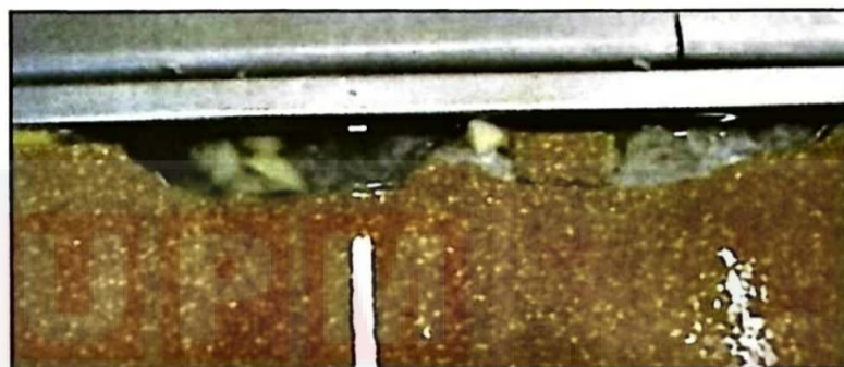
Figure 2.6 1 Poor floor-to-drain interface installation that can harbor microbial growth (EHEDG Doc 44, 2018)
